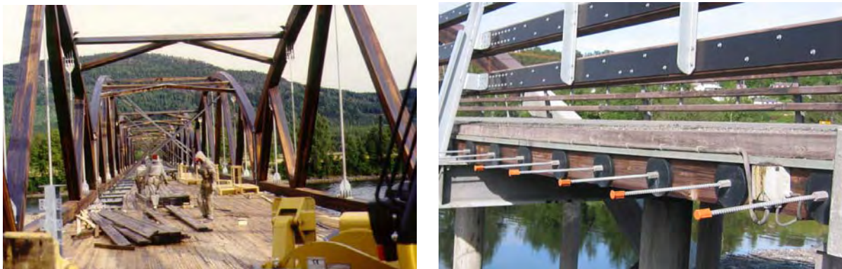
Fig. 15.12 Laying the deck of Evenstad bridge (photo: Moelven Limtre) and detail of Måsør bridge (photo: K. Bell)
