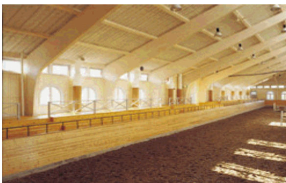
Fig. 5.12 Portal frame in a riding school (Reproduced by permission of Svenskt Limträ AB)
