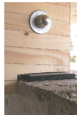
Fig. 18 Support of the roof elements at the end of the reinforced concrete wall
