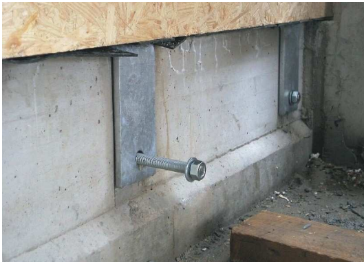
Fig. 15 Connection of the wall element with the foundation by means of steel angles
