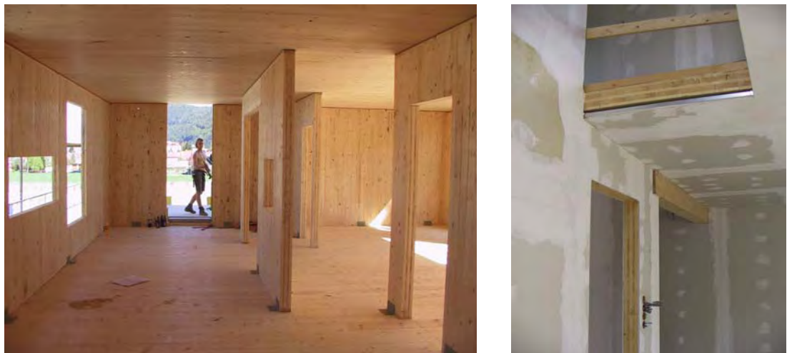
Fig. 31 Load-carrying elements and shear-walls in a multi storey building; floors with openings
