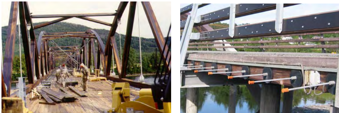
Fig. 12 Laying the deck of Evenstad bridge (photo: Moelven Limtre) and detail of Måsør bridge (photo: K. Bell)
