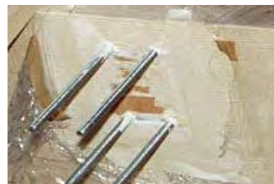
Glued-in rods (loaded transversal to their axis)
