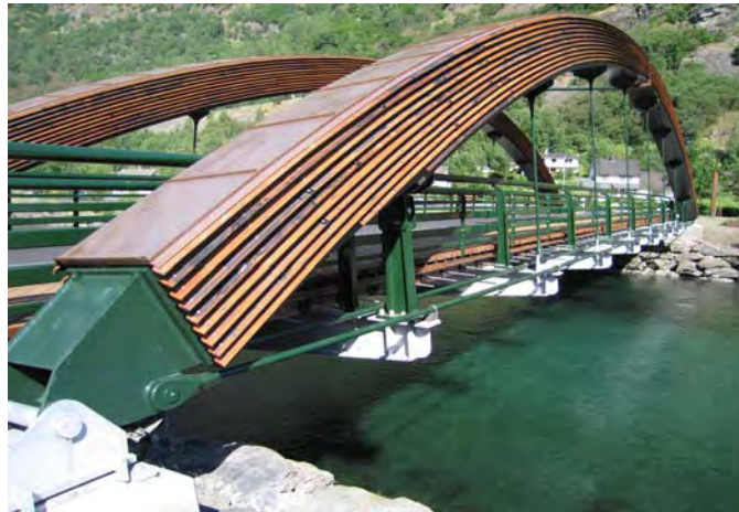
Fig. 17 Fretheim bridge at Flåm in western Norway (photo: R. Abrahamsen, SWECO Grøner AS)
