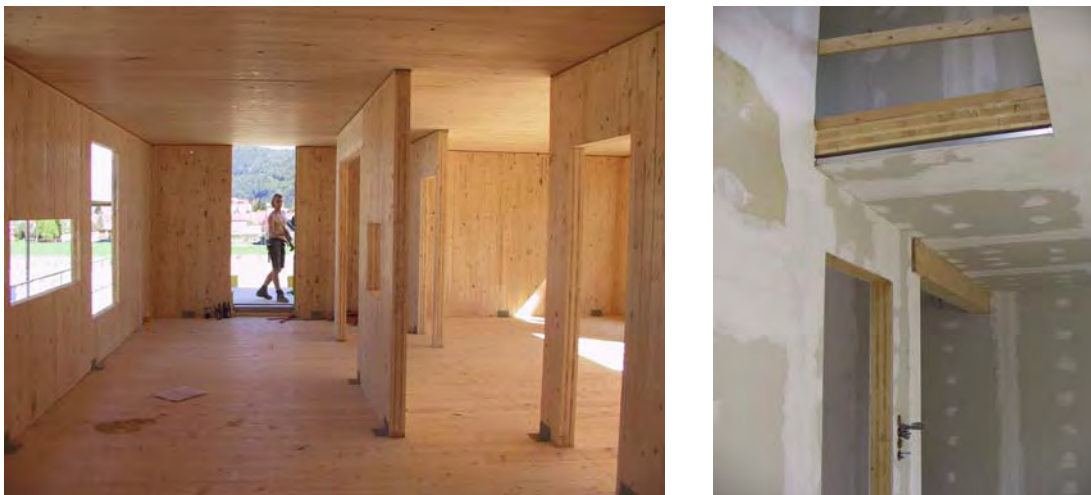
Fig. 30 Load-carrying elements and shear-walls in a multi storey building; floors with openings
