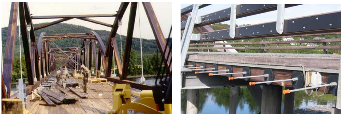
Fig. 12 Laying the deck of Evanstad bridge (photo: Moelven Limtre) and detail of Måsør bridge (photo: K. Bell)
